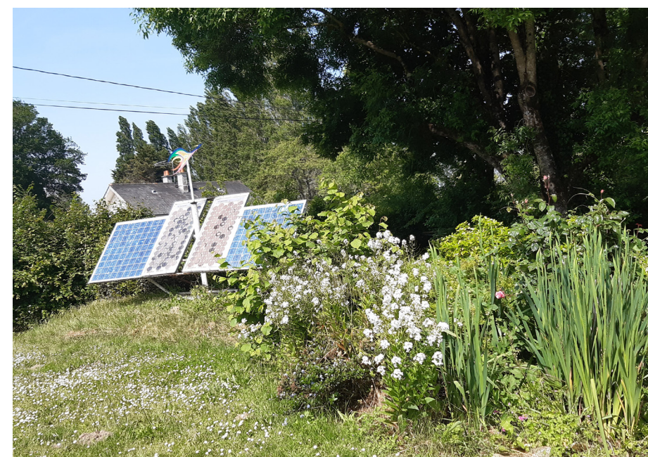
Photo-voltaic energy system
